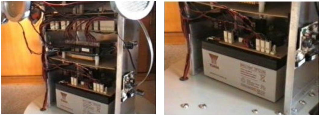
Figure 13 Frame where the PCBs are stacked
